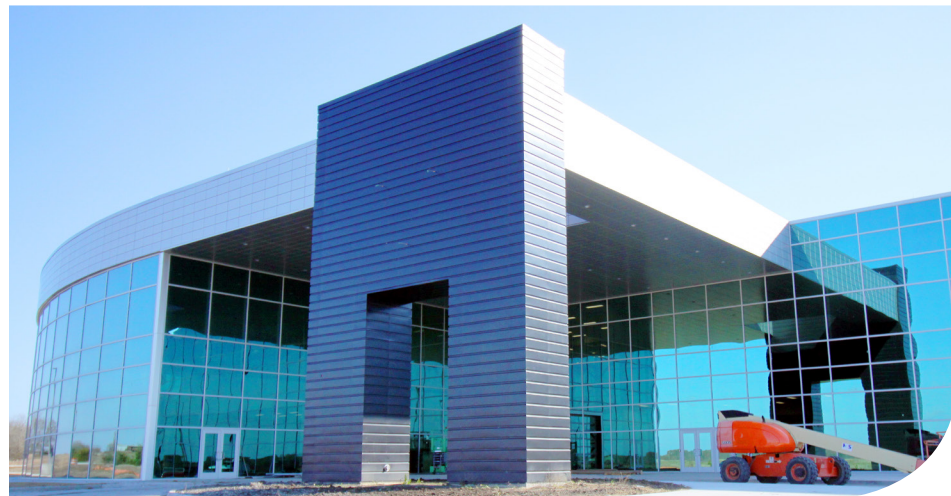
East Mississippi Community College's Center for Manufacturing Technology Excellence 2.0, or Communiversity, is expected to open to students in the fall of 2019.
